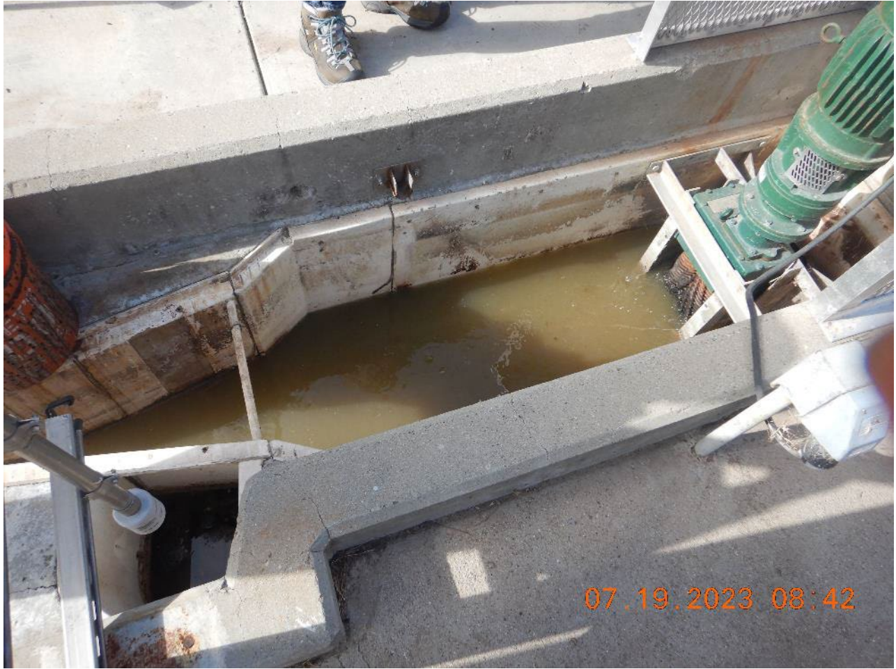
Photo 1. Influent stilling well with ultrasonic flow meter and an in-channel comminutor.
